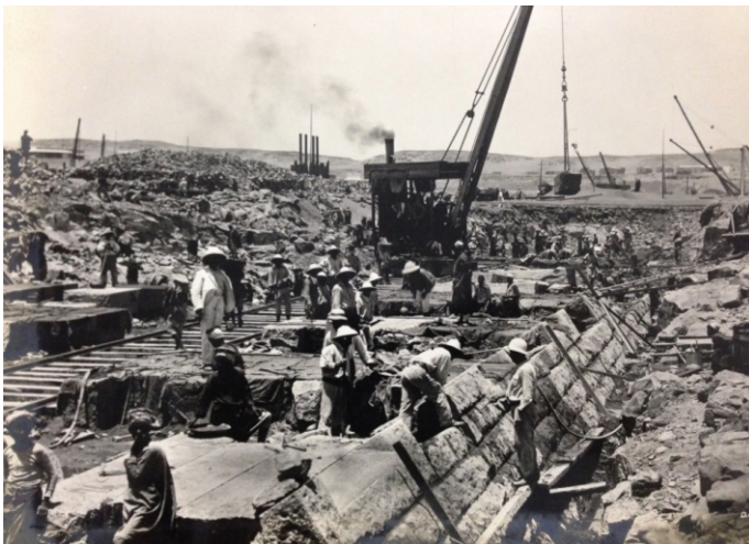
Photograph of Aswan Dam under construction (Reproduced from the photograph available with the Archival Section of Mahatma Gandhi Central Library, I.I.T. Roorkee)
